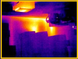
Poorly Insulated Walk-In Cooler
