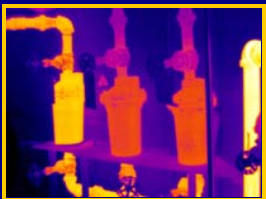
Leakage from a Steamtrap
